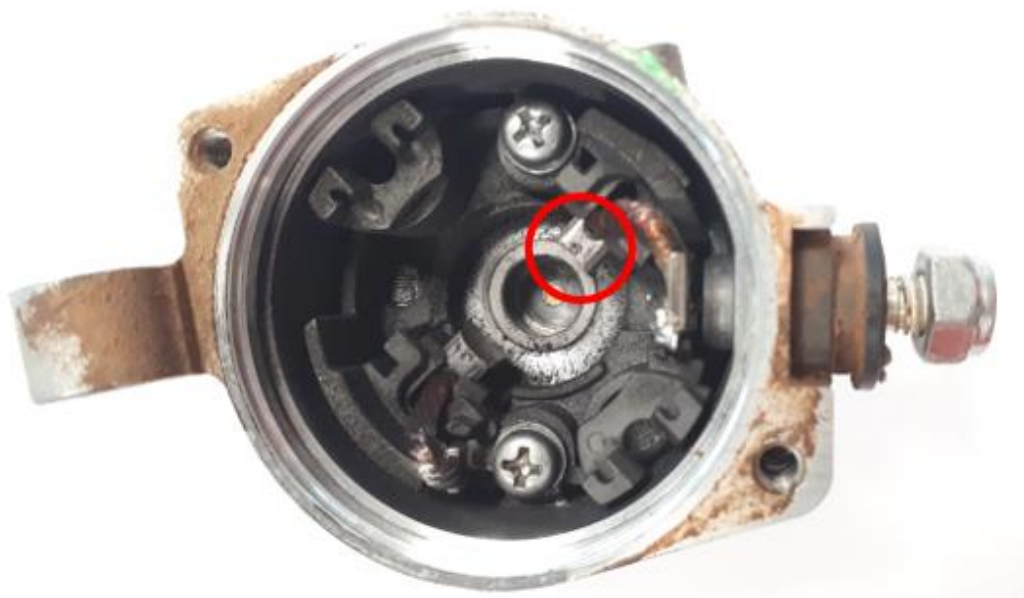
Brushes in poor condition
